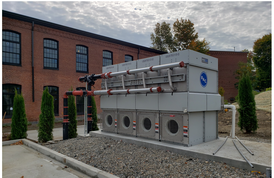
A historic mill building converted to residential housing. Heat pumps are used for heating and cooling.
